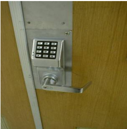
Door Cipher Lock installed
