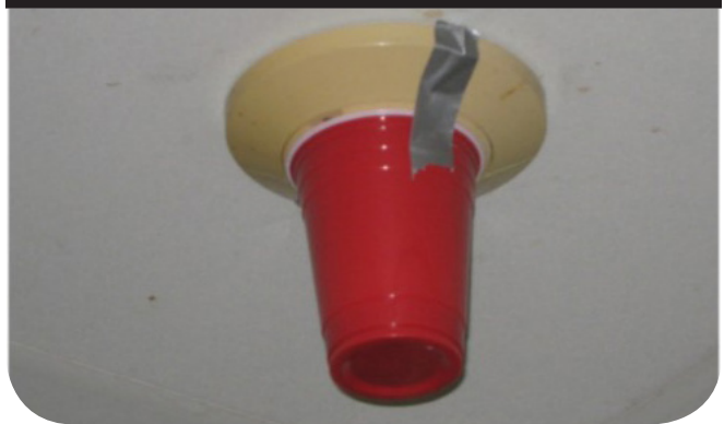
Covered Smoke Detector
