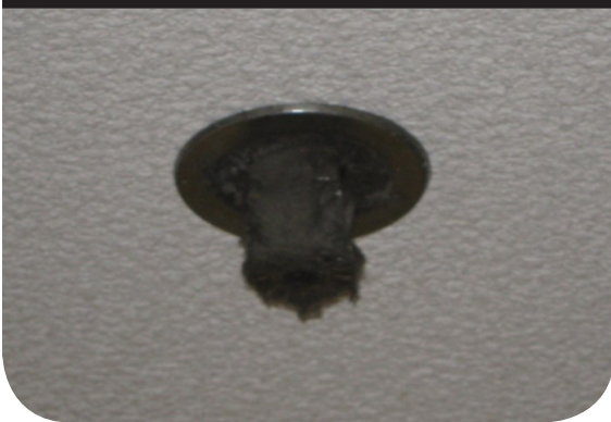
Dirty Sprinkler Head
