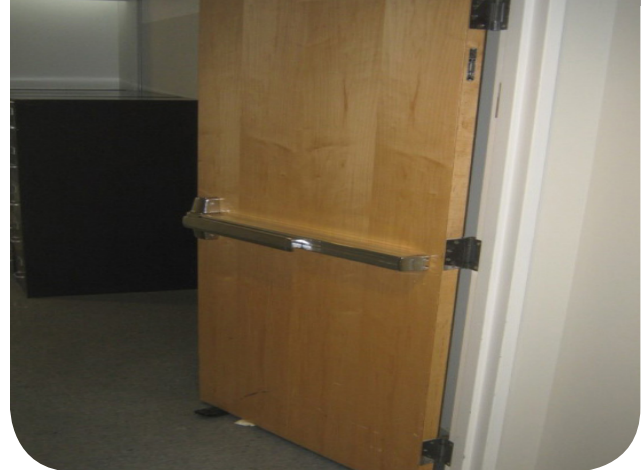
Propped Fire Door
