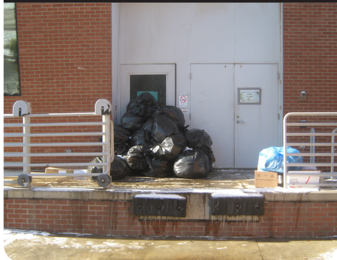
Blocked Exit Door
