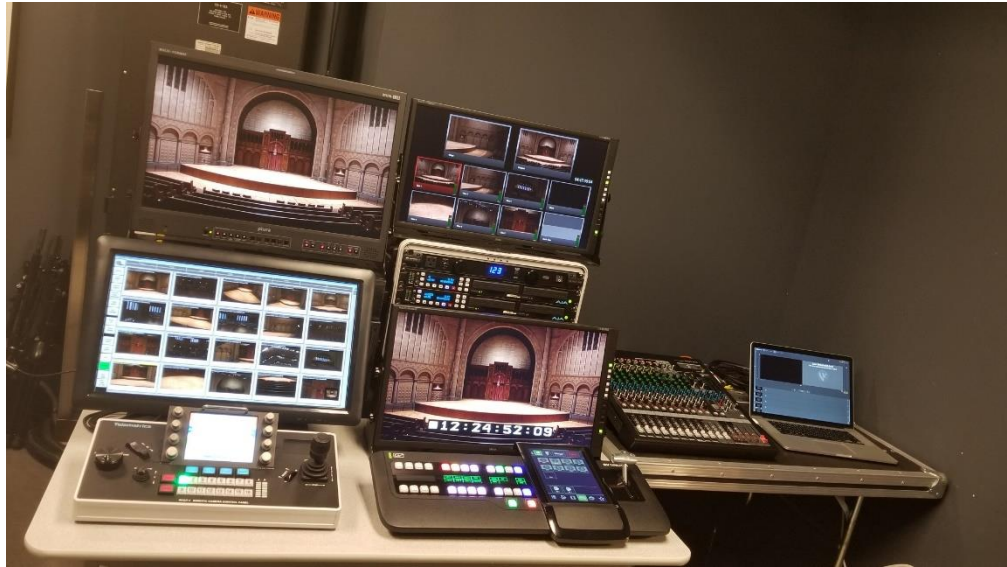
Extensive video recording system located in the A/V control room of Silver Hall
