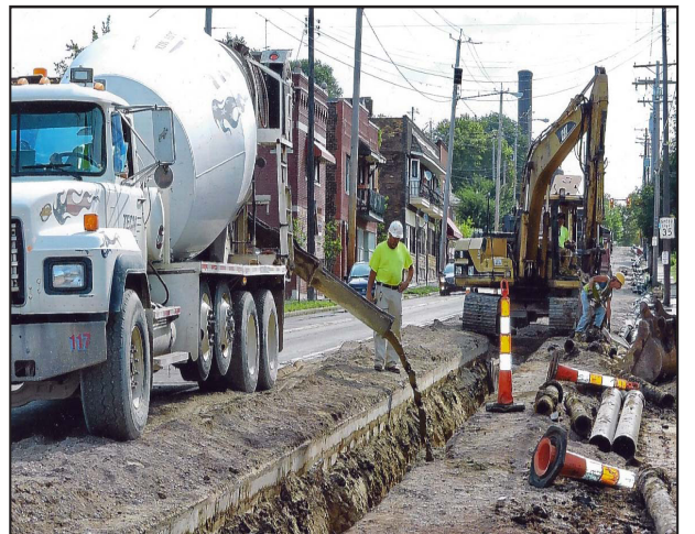
Utilicon Construction workers began resurfacing Woodland Avenue between E. 89th Street and Martin Luther King Jr. Boulevard in July with a May 2016 completion date for the $4,609,440.00 project. Traffic will be maintained with one lane in either direction during construction.
